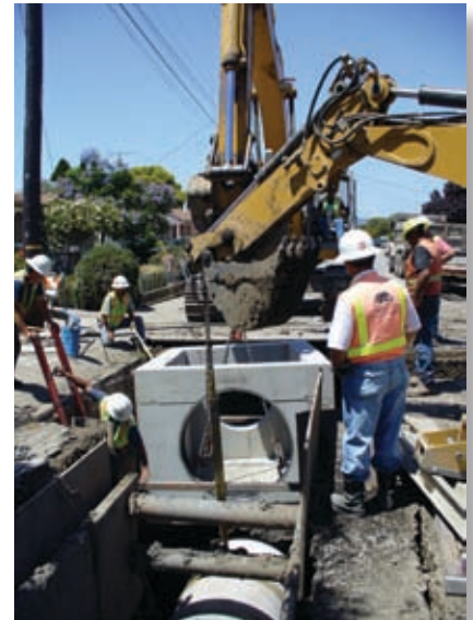
Photo right: Inspector monitoring the installation of a manhole at Swenson and Alexandria Streets.
