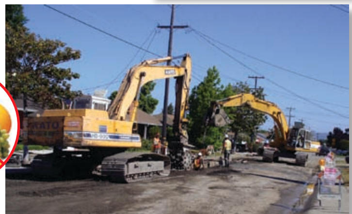
Photo below: Excavators installing 48-inch pipe and compacting subgrade on Swenson Street.
